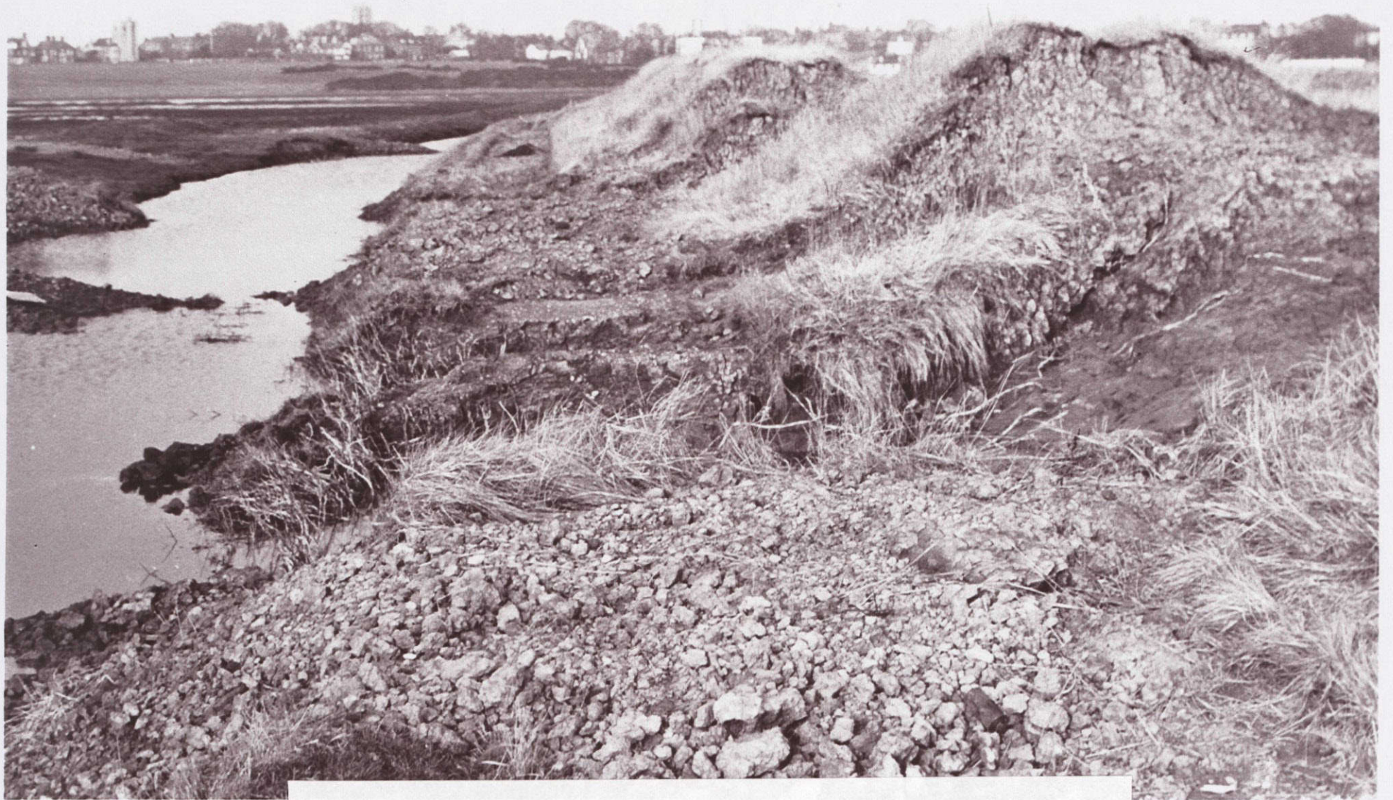
The Ferry footpath to Southwold, the sea has torn through the clay bank and spread the residue on the other side of the ditch.
